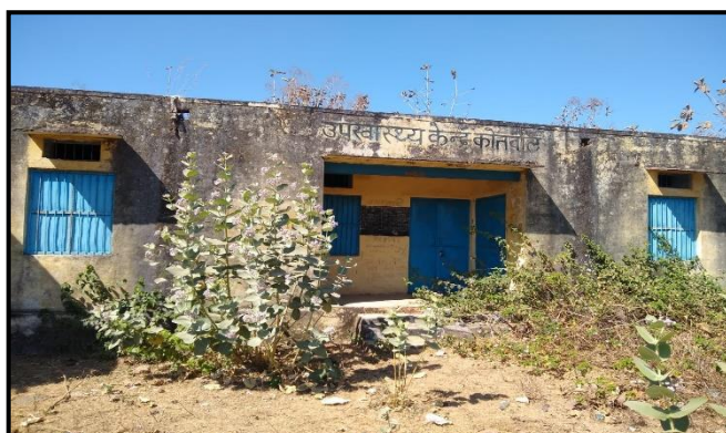
Before condition of sub-centre (Non-functioned from last 5 years)
